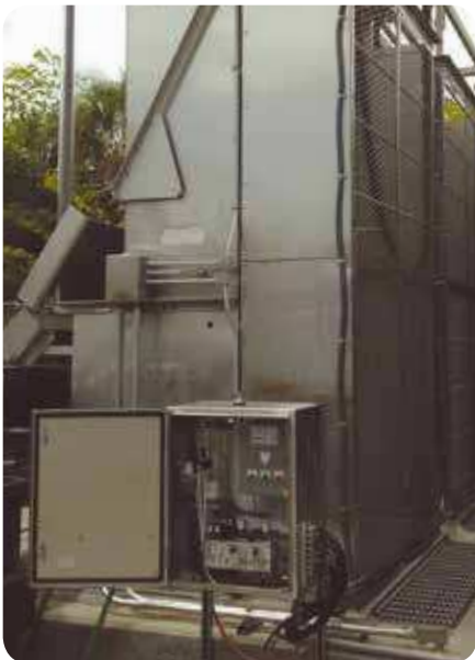
Waste water treatment
